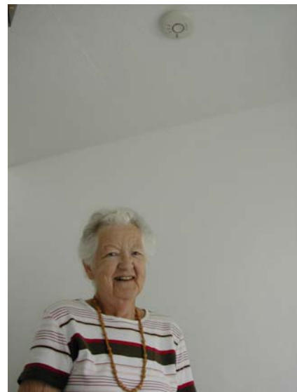
Mrs Brennan with her adapted Wi-Safe smoke alarm installed in her hallway
